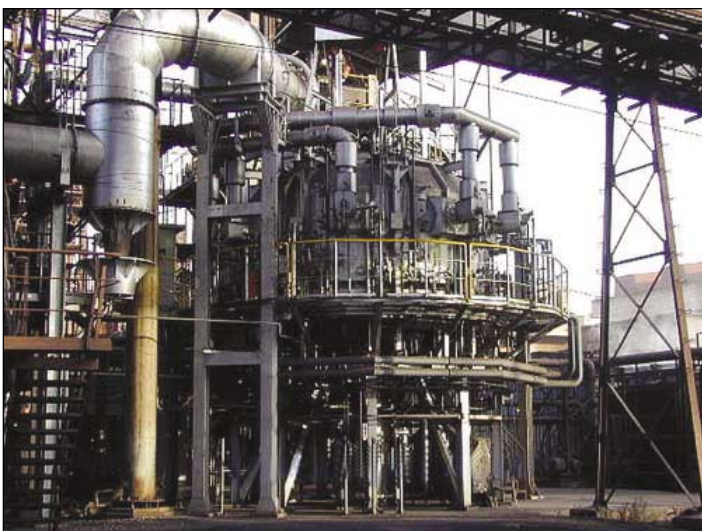
Figure 2 - ITmk3 Plant at Kakogawa Works
